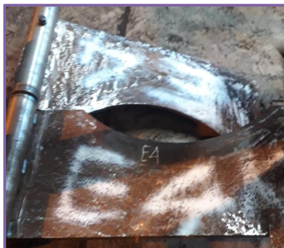
Figure 3. Visual Condition of Mechanical Orifice Before Maintenance
